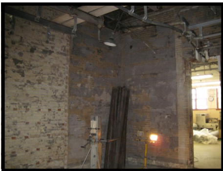
Interior walls in the carcass cooler on the second floor. Both freezers were removed in preparation for installing a large carcass cooler module and a freezer along the east wall.
